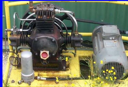
SynGas compressor (200 bar)
